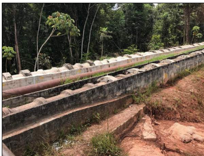
Figure 4.14 Effluent pipes in Area 45, steel pipe from DRS2 shown in the middle
