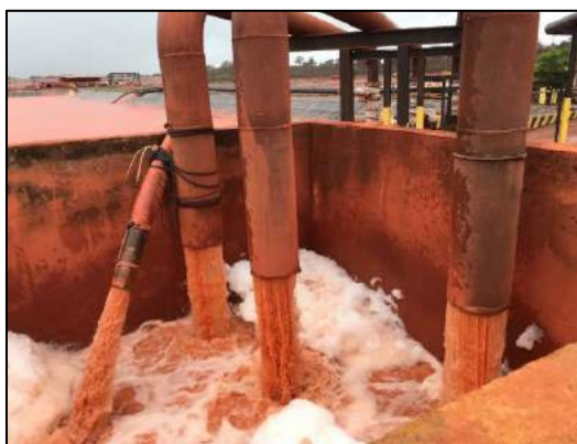
Figure 4.12 Effluent box in DRS1 showing permanent and mobile pumping into the box
